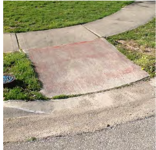
Example of +1/2" displacement at gutter line and horizontal displacement at top of ramp
