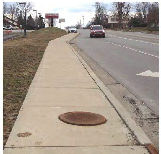
Example of displacement at utility
