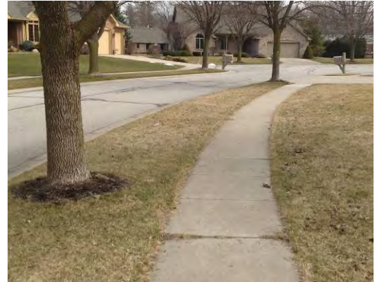
Example of displacement of sidewalk at tree
