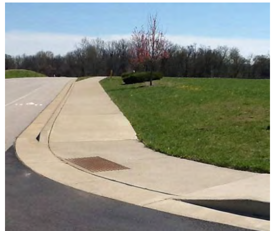
Example of DW that does not extend full width of curb ramp
